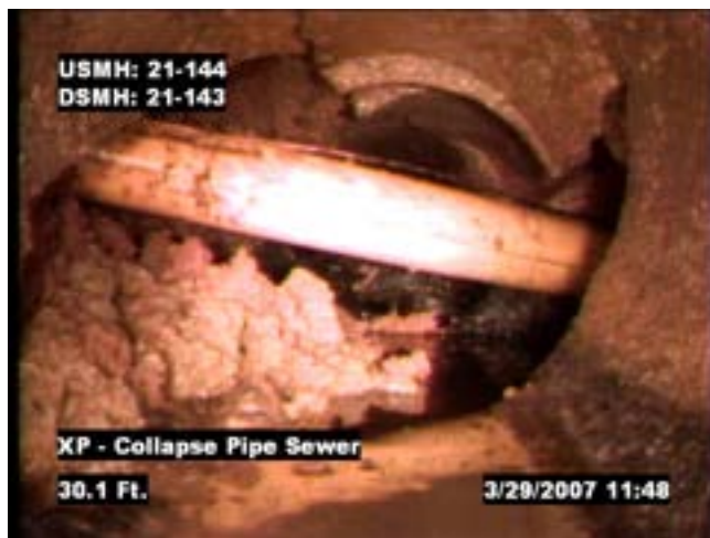
Fig. 1. Cross-bore of a natural gas distribution line in a sewer service lateral
