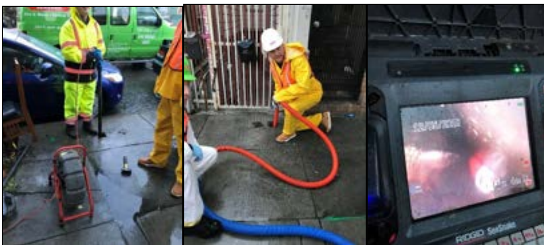
Figure 12 (left-right)—Inspection crew inserts optical camera at curb cleanout. ServPro crew inserts WET at property line cleanout. Real-time view of optical camera screen showing water being extracted.
