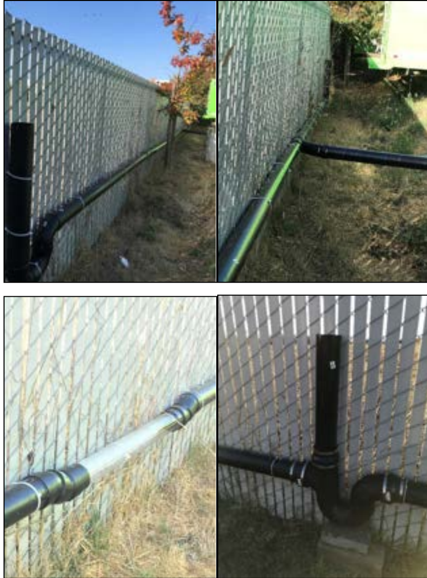
Figure 8 (clockwise)— Foundation access. Branch in sewer lateral. Curb access with p-trap. Sag in sewer lateral using clear PVC for viewing water extraction in progress.
