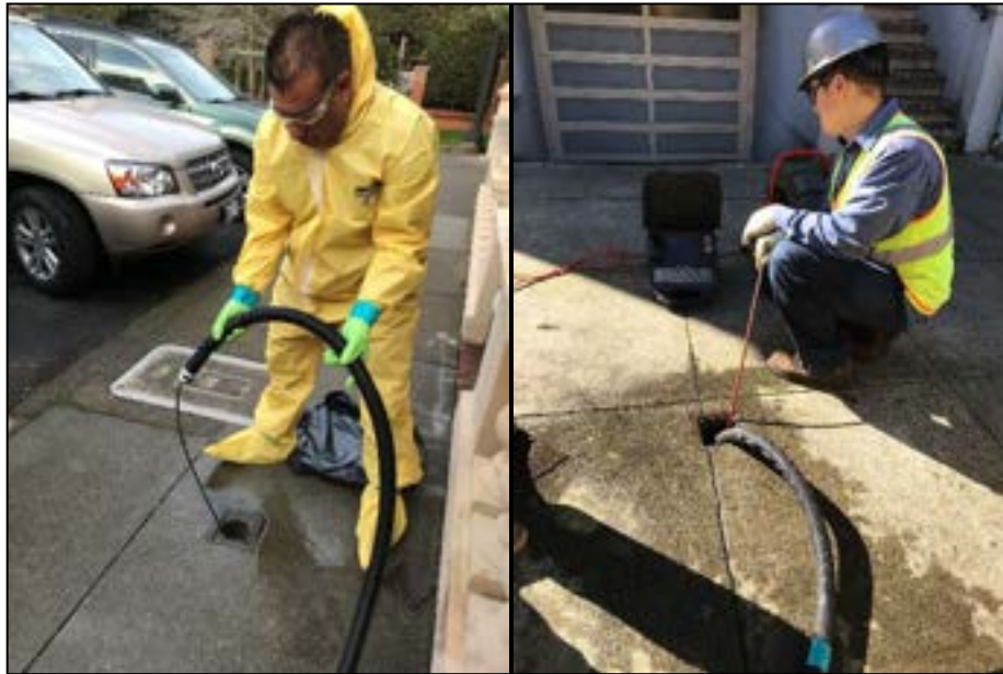
Figure 13 (left-right)— Plumber’s snake modification to the hose to assist with p-trap navigation. Water extraction and camera inspection occurring simultaneously at a multifamily complex.
