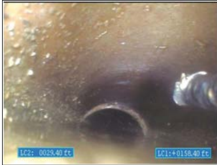
Figure 6—Example of water at the base of the interior of a sewer lateral as viewed by an inspection crew's camera.
